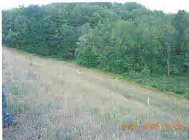
Detached earth embankment downstream slope
