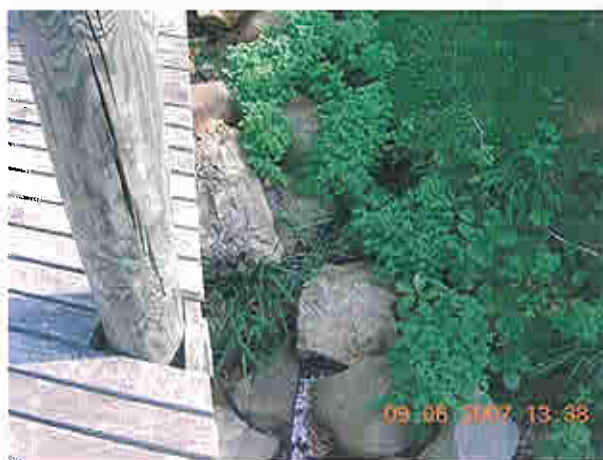
Riprap and seepage at left embankment of principal spillway
