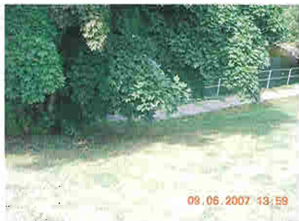
Downstream slope at principal spillway, left end, note large tree
