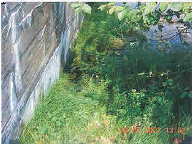
Seep at original spillway structure, left abutment wall
