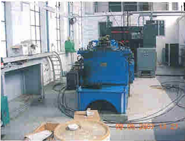
Interior of powerhouse
