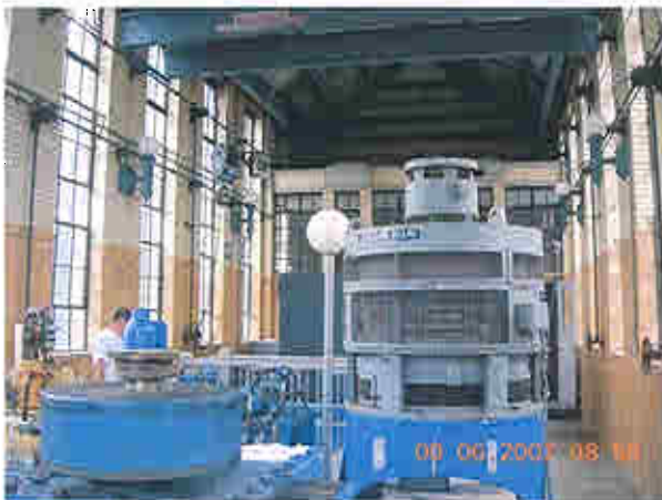
Interior of powerhouse
