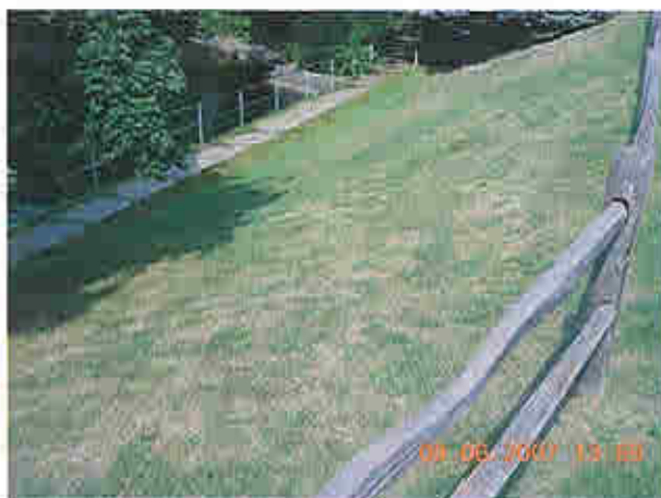
Downstream slope at principal spillway, note irregularities in slope
