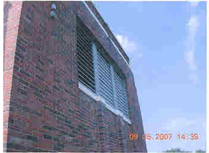
Right side of power house, note corrosion of window framing Failing brick work noted
