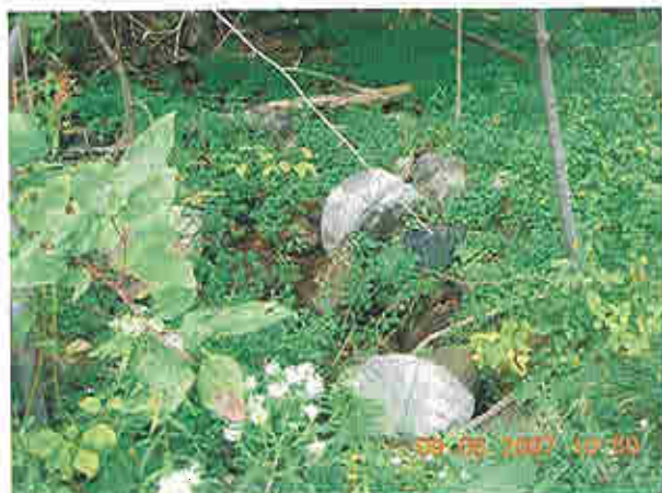
Seepage at left end of detached earth embankment
