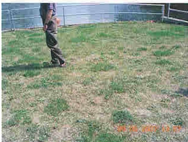
Left end of upstream slope at principal spillway, irregularities In slope noted
