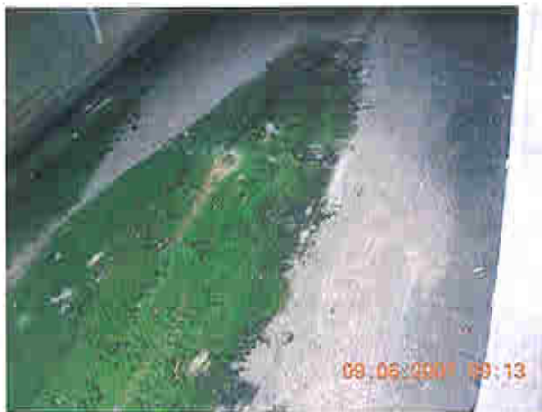
Downstream of spillway, note seepage
