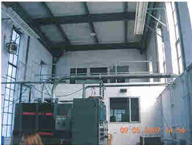
Interior of power house, note make-shift roof leak collection
