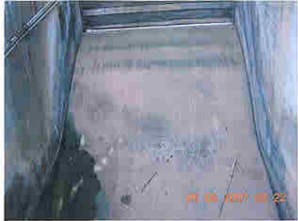
Downstream side of spillway, note seepage
