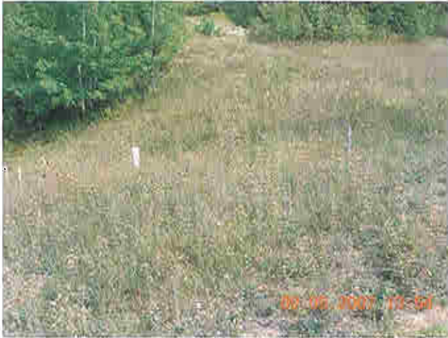
Downstream slope of right embankment- note, piezometers (County continues to monitor piezometers)
