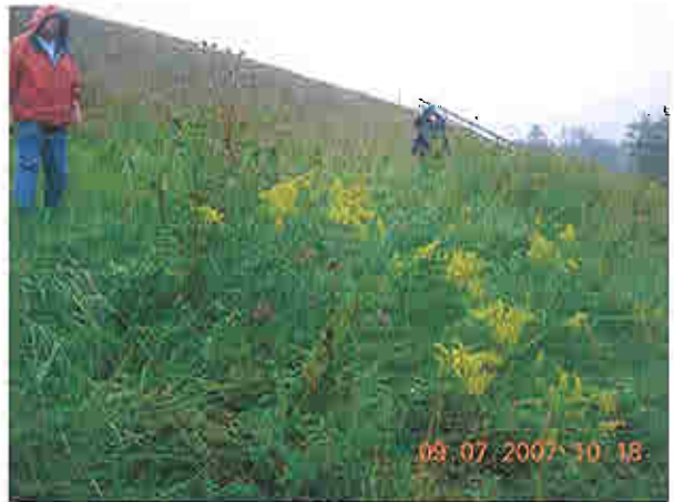
Downstream slope of right embankment, note heavy vegetation near bottom quarter of slope
