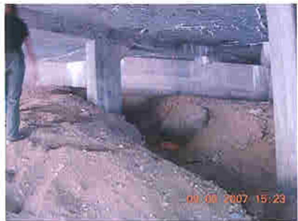
Underneath access deck, note cracking and deterioration
