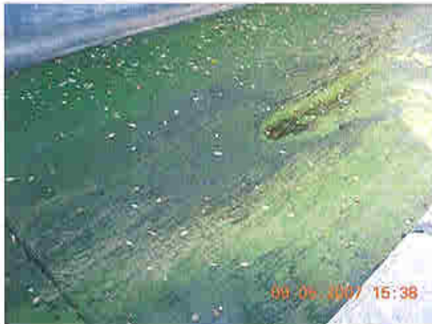
Downstream of spillway, note seeps in bottom of channel
