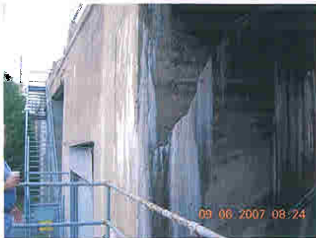
Right wall at spillway, note cracks
