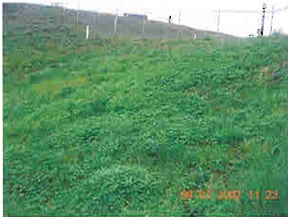
Downstream slope of left embankment, note vegetation, irregular ground surface noted, some soft areas
