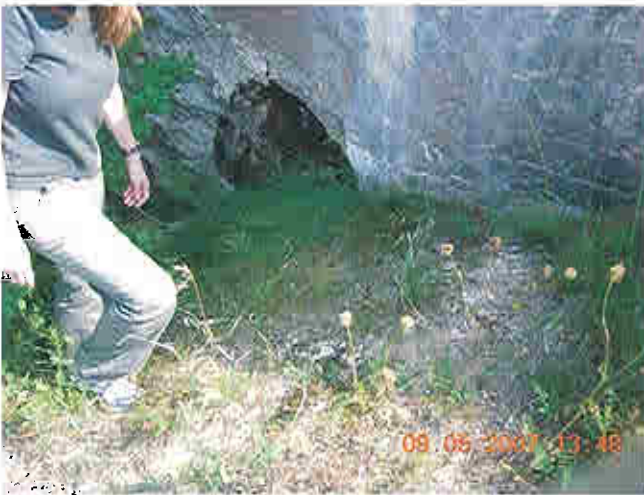
Seep at original spillway structure, right abutment wall
