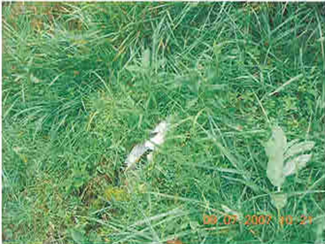
Pipe with flowing water and sedimentation, downstream slope of right embankment
