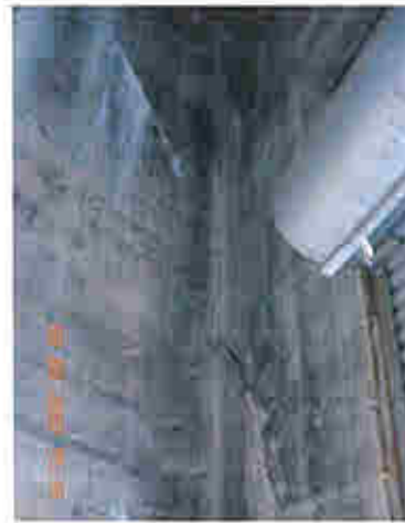
Storage bay, note cracks
