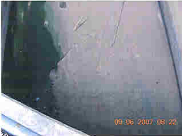
Downstream side of spillway, note seepage
