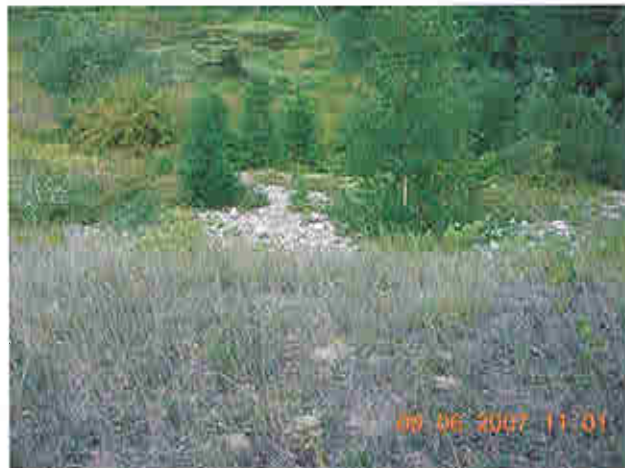
Downstream of detached embankment, note stone
