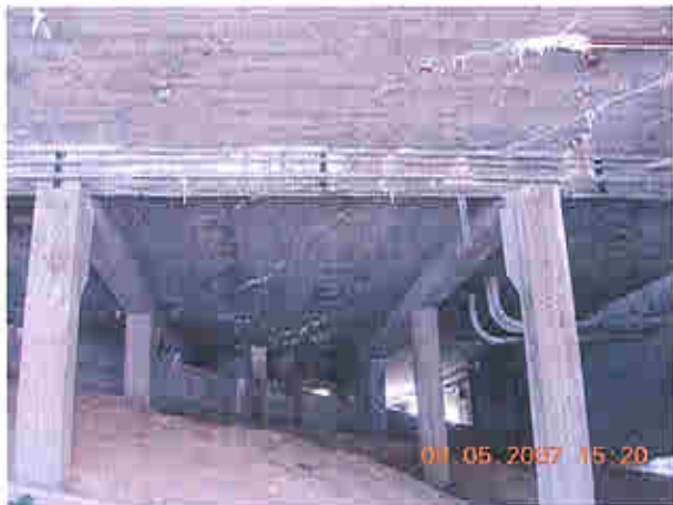
Underneath access deck, note cracking and deterioration
