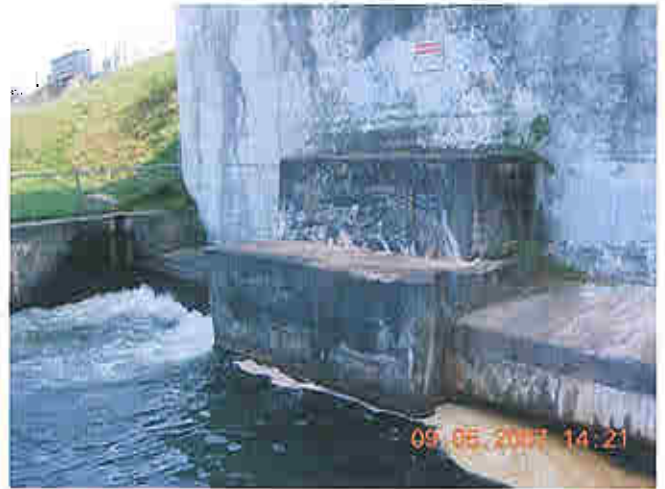
Downstream side of powerhouse, view from left embankment, note spalling/ deterioration
