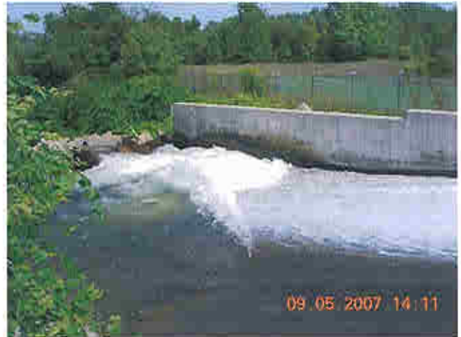
Downstream of stop log and tainter gate spillways, view from intermediate embankment, looking right
