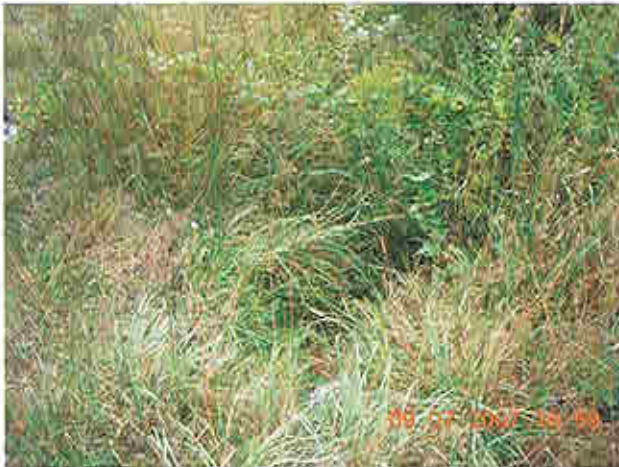
Seepage downstream of downstream slope of right embankment
