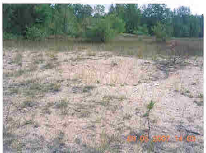
Downstream of right embankment, unvegetated sandy area with unexplained hole
