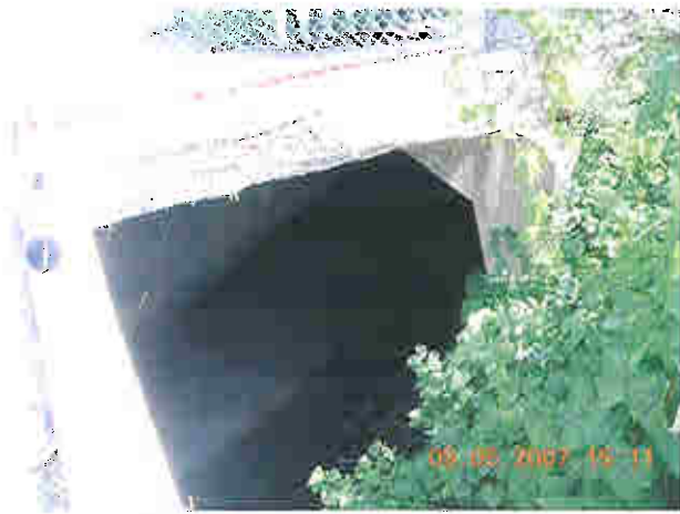
Access deck to the left of the powerhouse, note deterioration
