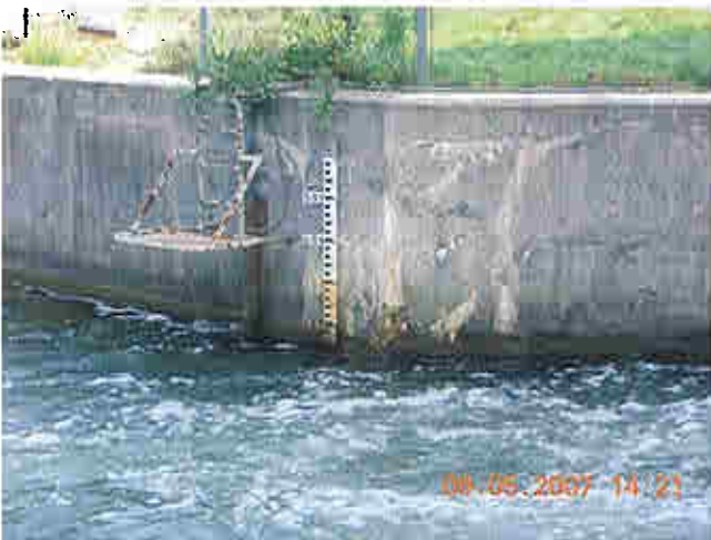
Tail water staff gauge downstream of power house (County reads head and tail water elevations each day)
