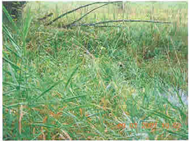
Stream downstream of downstream slope of right embankment assumed to originate from seepage at slope
