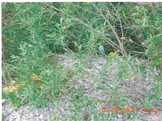
Downstream of detached embankment, note stone and pipe
