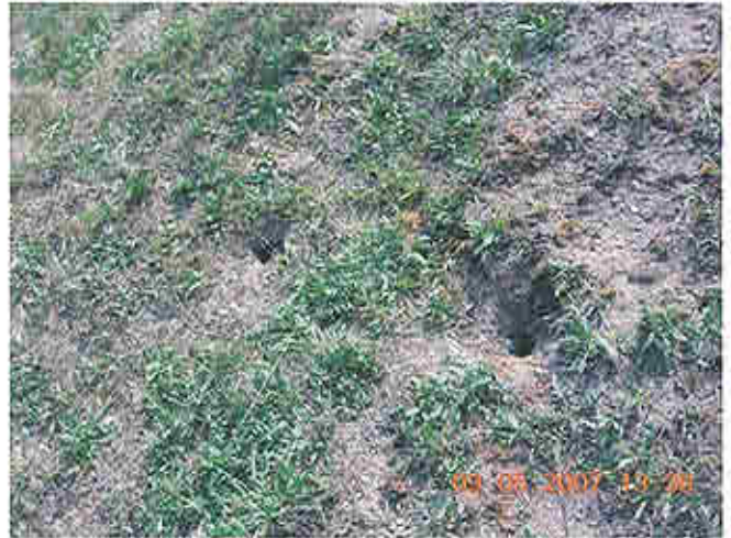
Rodent holes observed at downstream slope of intermediate embankment
