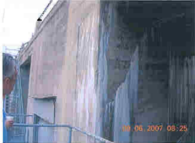
Right wall at spillway, note cracks
