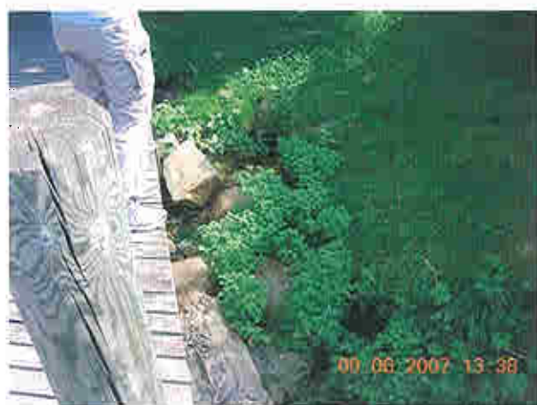
Riprap and seepage at left embankment of principal spillway
