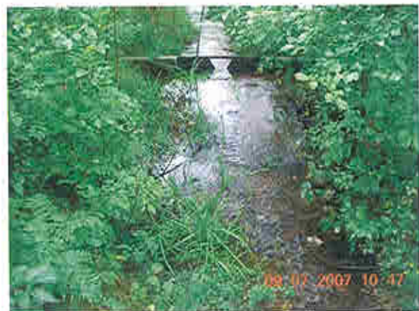
Monitoring weir downstream of downstream slope of right embankment- assumed to measure seepage flow
