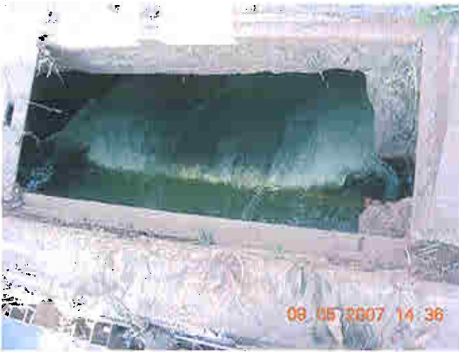
View looking down at stop logs at power house spillway, concrete deterioration noted.
