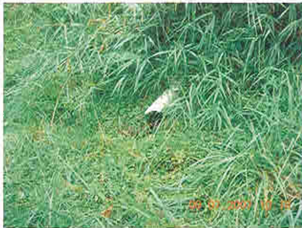
Pipe at downstream slope of right embankment
