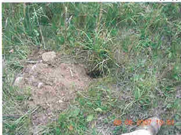
Rodent hole on downstream slope of detached embankment
