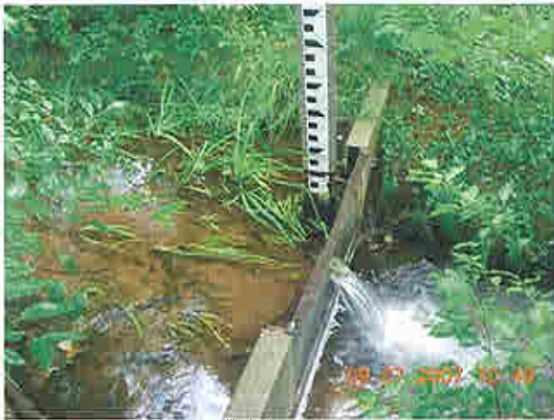
Monitoring weir downstream of downstream slope of right embankment- assumed to measure seepage flow
