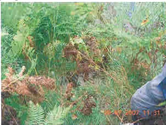
Downstream slope of left embankment, note heavy vegetation, erosion noted along fenceline
