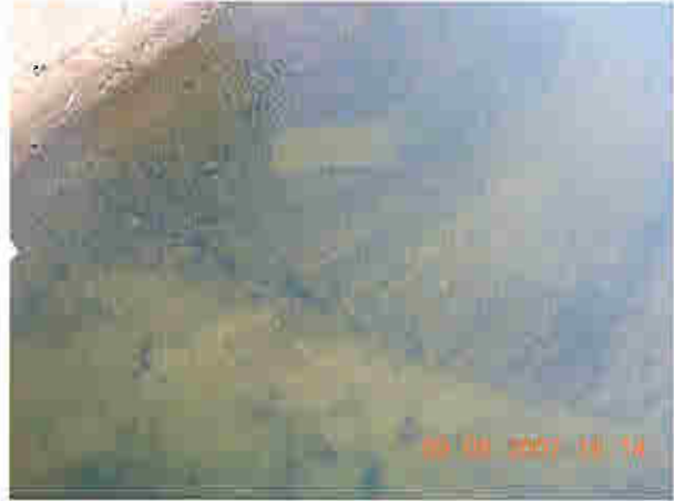
Upstream of road and intake, note possible concrete debris
