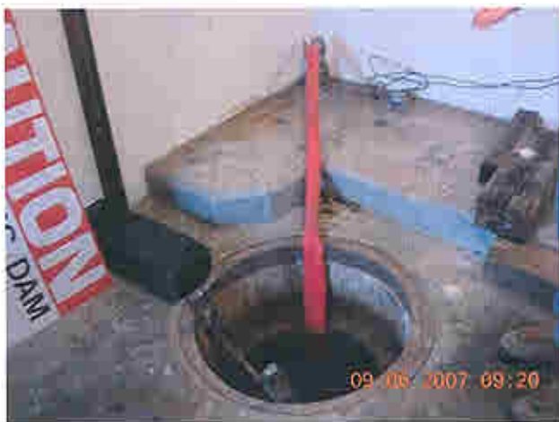
Lower level of powerhouse, location of "leak" earlier this year
