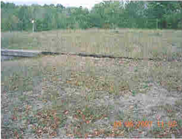
Sheet pile extending at right side of concrete wall at detached embankment
