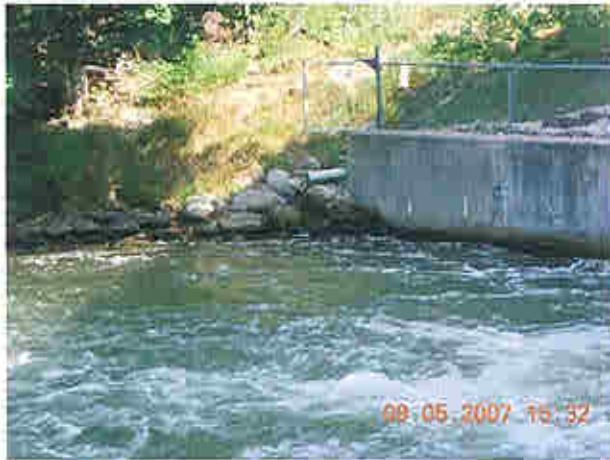
Right downstream abutment of powerhouse, note water flowing
