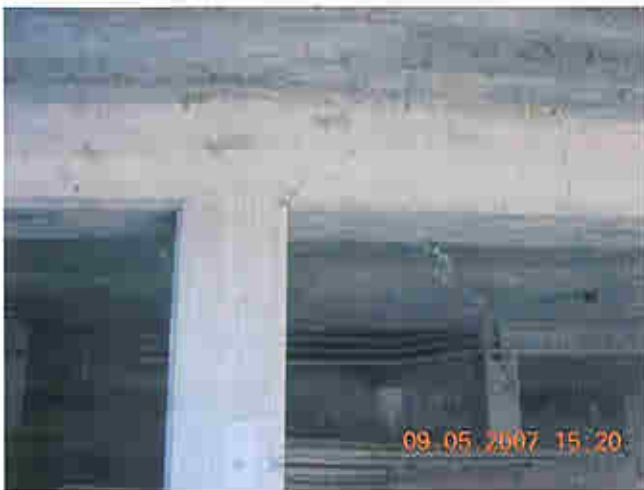
Underneath of access deck, note cracking and deterioration
