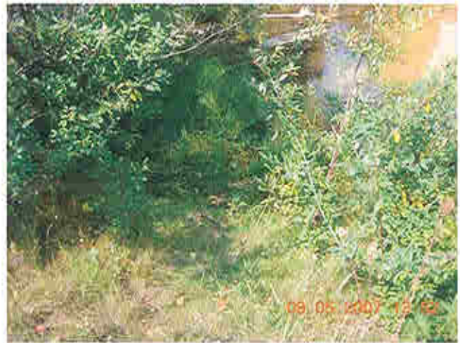
Seep at toe of right embankment, near standing water
