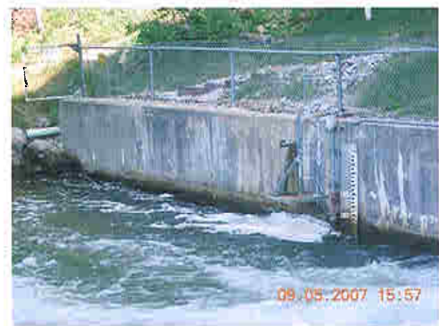
Right side downstream of powerhouse
