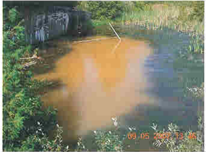
Standing water downstream of right embankment (downstream of original spillway)
