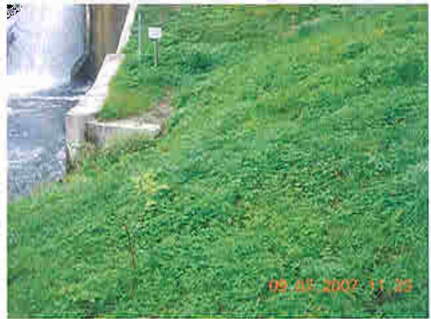
Downstream slope of left embankment, note vegetation, irregular ground surface noted, some soft areas
