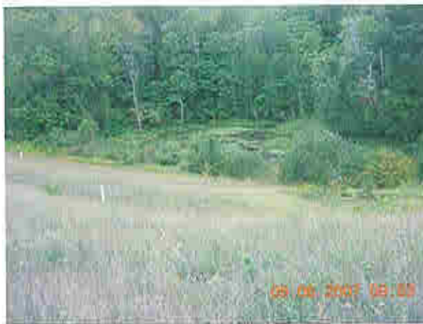
Detached earth embankment, downstream slope, note standing water at toe of slope
