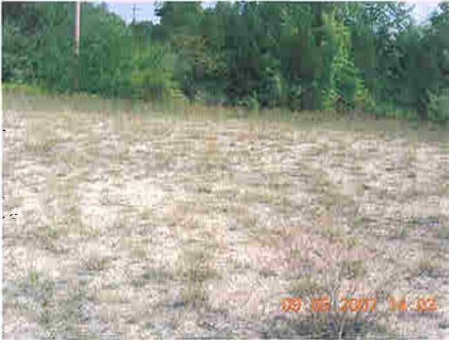
Downstream of right embankment, unvegetated sandy area
