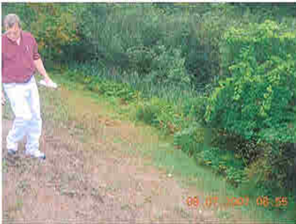
Downstream slope of left embankment at left end, note wet toe
