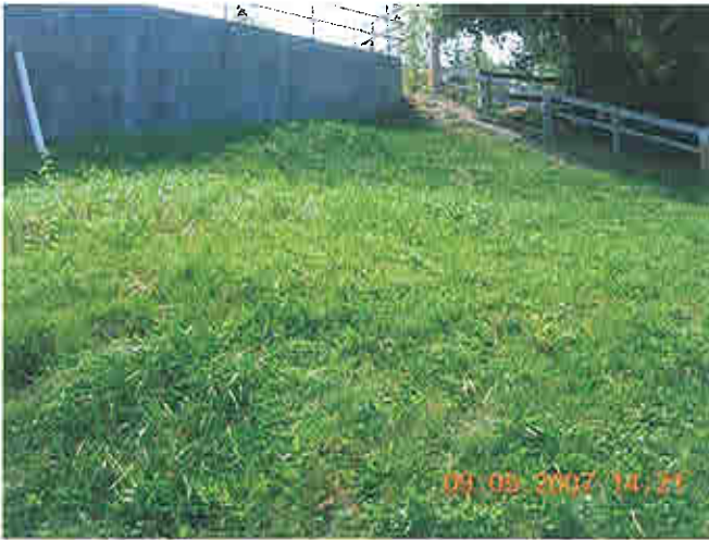
Downstream slope of left embankment, soft moist areas
