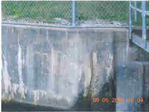
Right side downstream of spillway, note cracking
