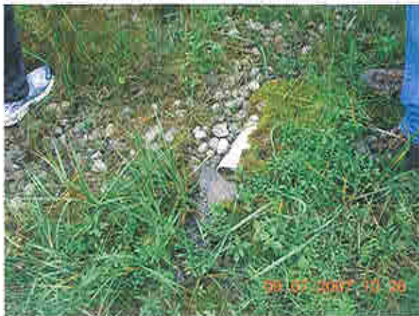
Pipe with flowing water and sedimentation, downstream slope right embankment
