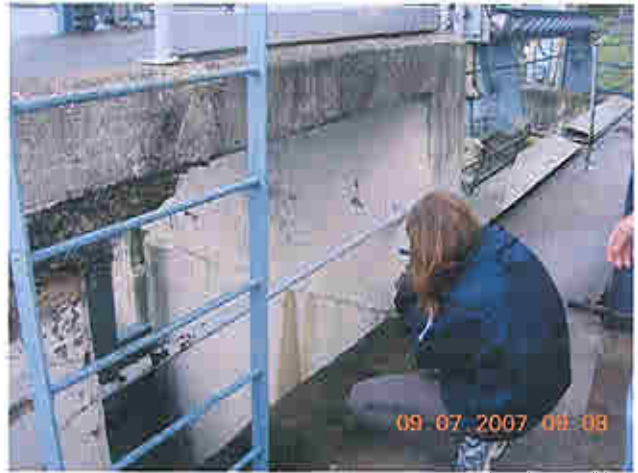
Support at tainter gate, note cracking and degradation
