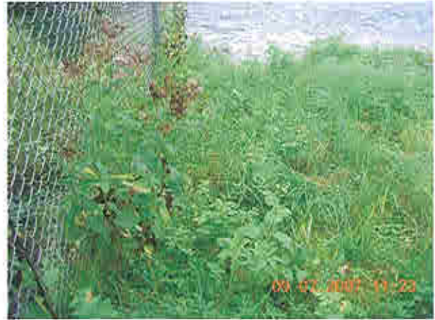
Downstream slope of left embankment, note heavy vegetation
