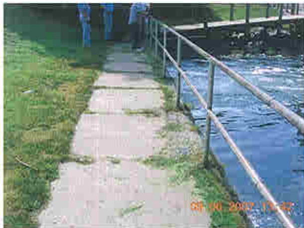
Sidewalk adjacent to downstream side of principal spillway Note seepage at edge of sidewalk
