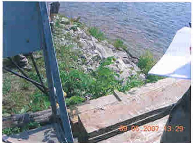
Upstream shoreline of the intermediate embankment- note rip rap placed to control erosion.
