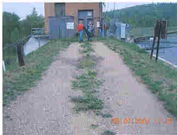
Roadway just left of powerhouse, view looking right Note low area in roadway
