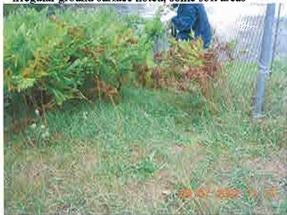
Downstream slope of left embankment, note heavy vegetation, erosion noted along fenceline
