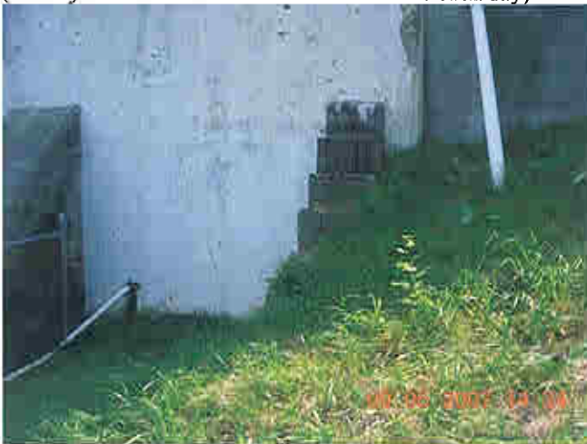
Area of seepage at powerhouse at left embankment
