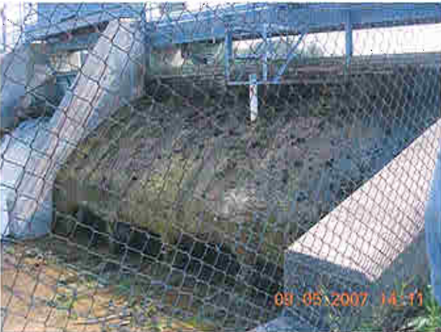
Downstream side of stop log spillway, note spalling/ deterioration
