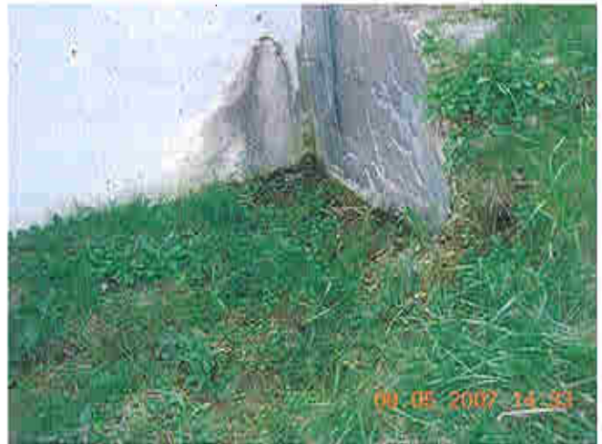
Seep at powerhouse at left embankment
